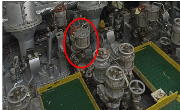
Figure 3. Main boiler FO piston valve
