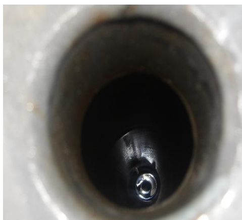
Figure 6: Empty De-aerating Tank
