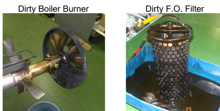
Figure 5: Burner & F.O. Filter Condition
