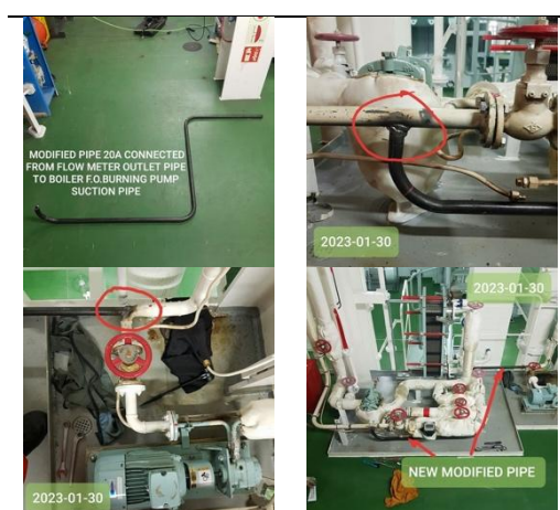
Figure 9: Results of modified boiler fuel oil pipe system Source: authors
